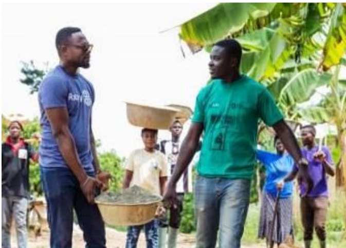
Cosmos Segbefia, a member of the Rotary Club of Sekondi-Takoradi, and Derrick Ababio Kwarteng, of Global Communities, assist with the construction of a borehole in the Western Region of Ghana in 2018. A report by Johns Hopkins University prepared for Rotary International estimated that Rotary members provide about 47 million hours of volunteer effort a year at an estimated value of $850 million.
